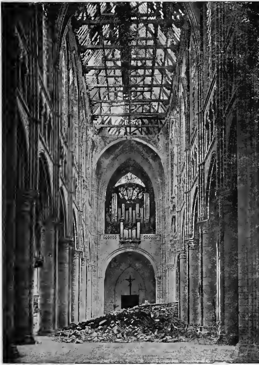
THE FALLEN VAULTING LEFT BAR: THE DAMAGED FRAMEWORK OF THE ROOF.
